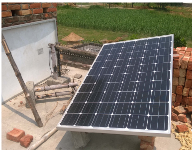
Figure: HPS Panel
